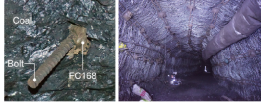
Fig. 7. Detailed show for fully bonded bolt (left) and photo for section supported by fully bonded bolts (right)
